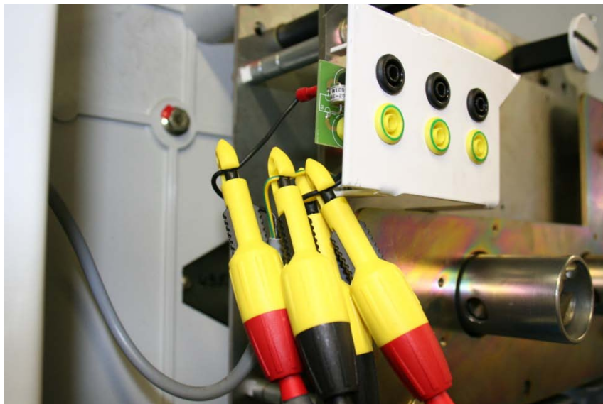
Figure 1: Earthing of the voltage indicator
