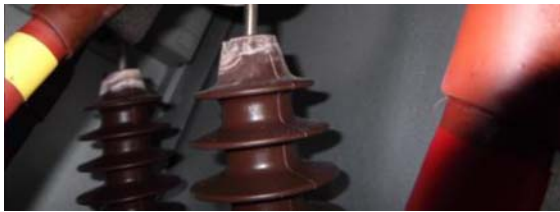
Figure 6: Degradation due to tracking after 12 years in service in normal service conditions
