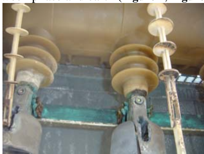
Figure 2: Degradation including tracking
