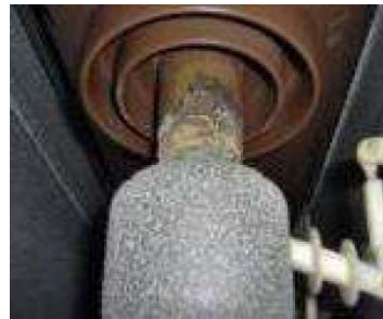
Figure 3: Degradation due to corona effect
