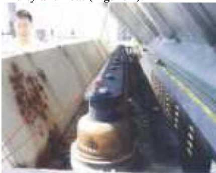
Figure 1: Corrosion on metallic part on a RMU
