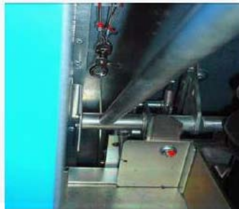
Photo 11: Operating handle in drilling space
